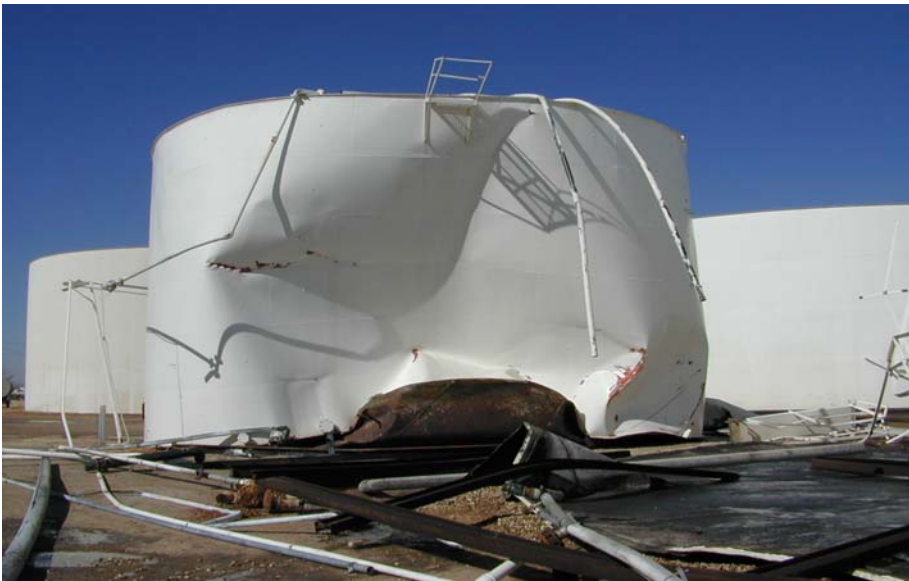
Figure 4. Damage to an adjacent tank caused by the impact of the unfurling wall of the failed tank.
