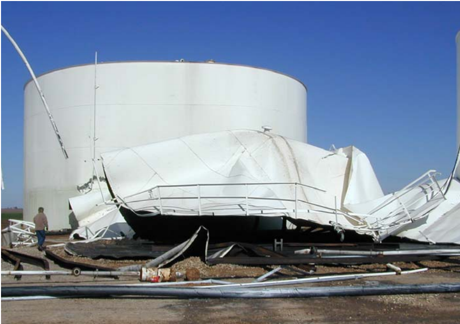
Figure 3. Failed liquid fertilizer storage tank.
